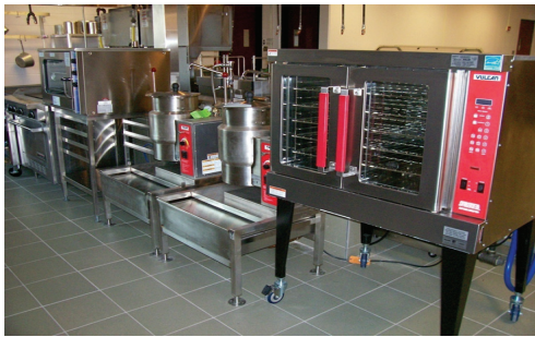
Figure 3: Back Line Kitchen Equipment Battery
